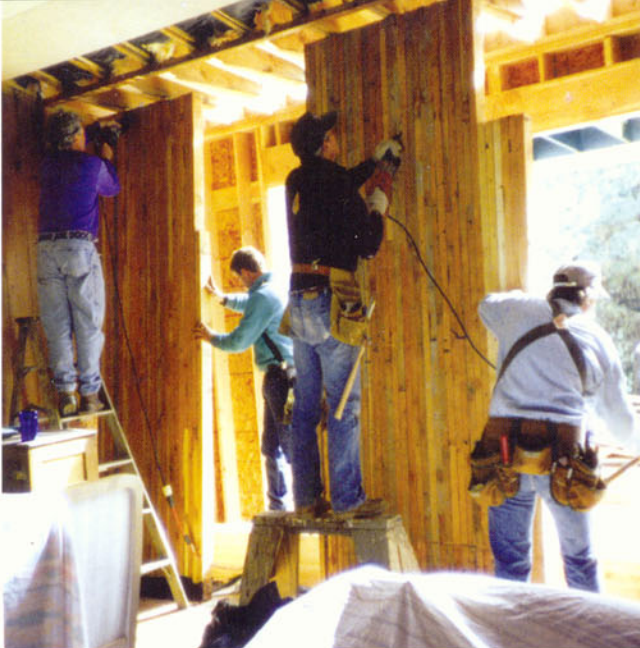
1994, tearing out the front wall of the house, hundreds of 2 x 4's were found behind the paneling.
